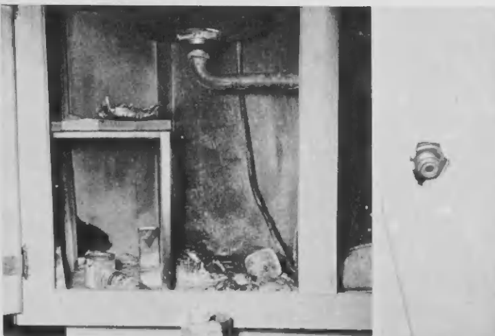
The impact of the explosion is visible in the lower left corner of the cabinet where a hole was left. At right, an identified flying object (can) landed in the ceiling.
